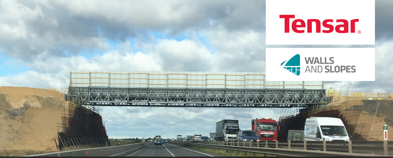
Three temporary bridges, supported on load bearing reinforced soil abutments built using Tensar's TensarTech TR2 system, allowed construction traffic to cross the busy A14, saving time and money.
