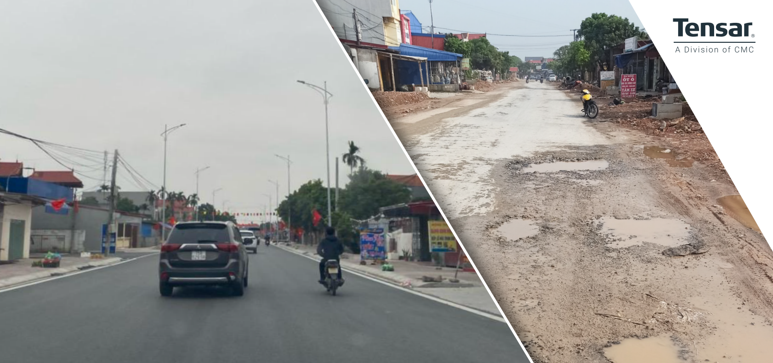
(Left) Highway construction completed in 2021 (Right) Damaged old pavement structure before reconstruction.
